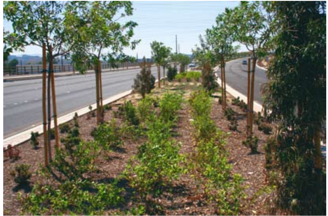
MOVING MOUNTAINS – There are not too many people who can say that a mountain was moved in order to install their project, but David Moralez can do just that, as a large hill was partially demolished to put the road through.
