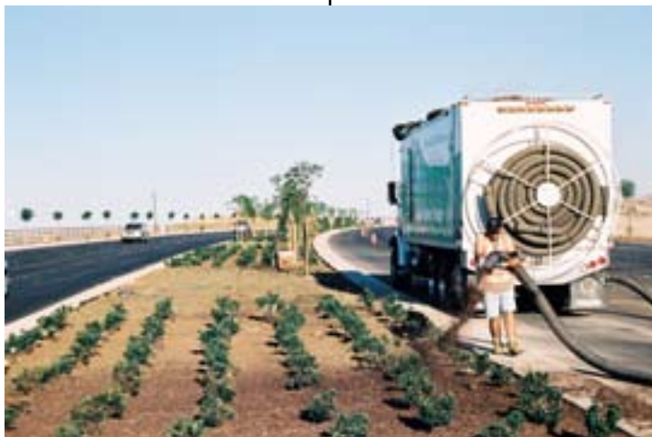
MULCH APPLICATION 101 – Move over sacks, wheelbarrows and rakes. Make room for a more efficient way of applying mulch bark...by blowing it in...all 1,000 yards of it.
