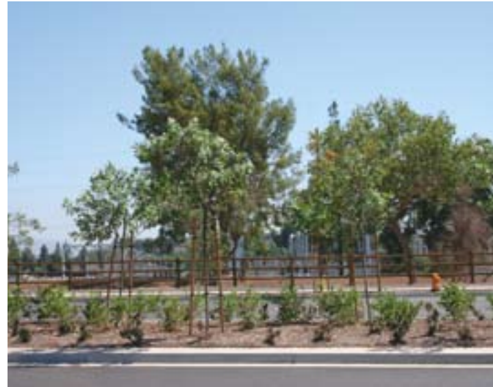
EXISTING TREES alongside the project are lonely no longer. That's because they are now joined by close to 1,000 trees installed by the Eco-Logic team at Cross Valley.
